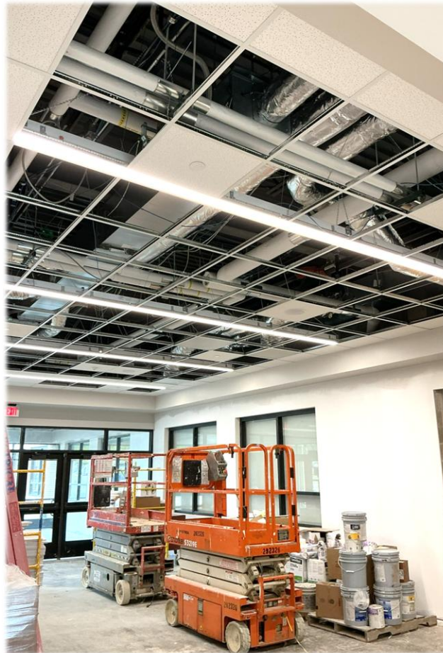
Commons Lighting and Ceiling
