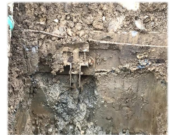
Existing Helical Pier
